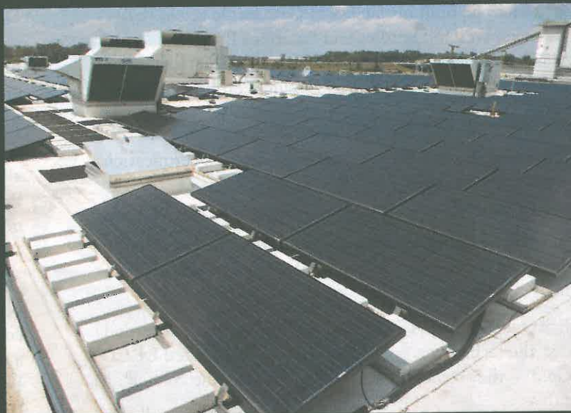
The solar panels on the roof account for 20 percent of energy used at Wetland Studies and Solutions, Inc.
